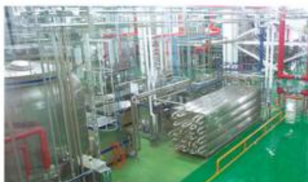
前處理設備 Pre-treatment equipment
